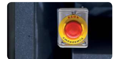
Emergency bell Automatic broadcasting using control inputs
